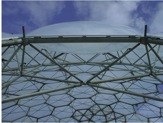
Fig. 16 The installed cushion
