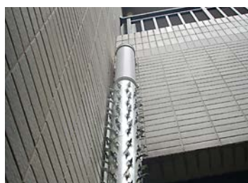
Razor spikes pipe school building.
