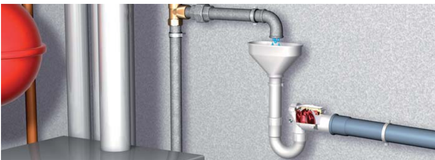
... furnace condensation overflow
